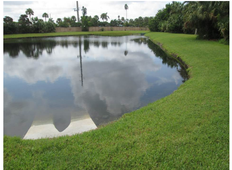
Pond 6 – 12" vertical erosion on north and east banks, add plants
