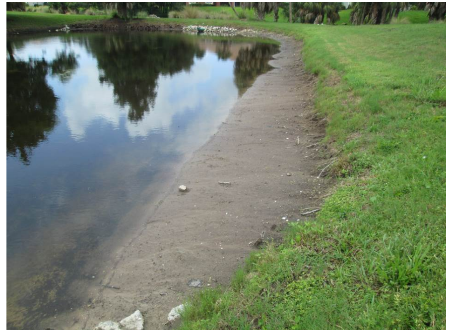
Pond 7 – 12”-18” of erosion along west side bank on north side
