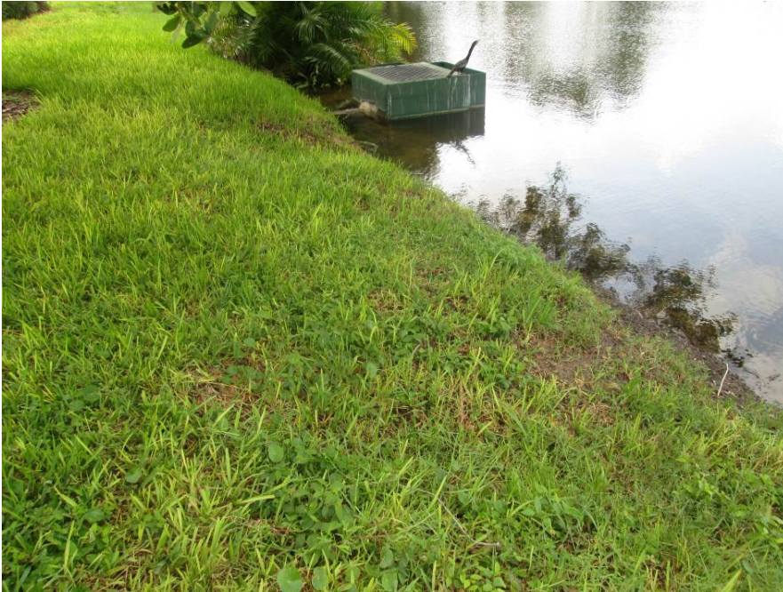
Pond 4 – Minor spot erosion on north side near west end
