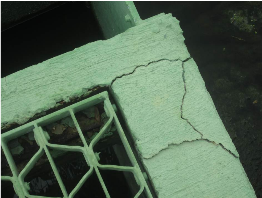
Pond 9 – Minor cracking on outfall control structure on southeast bank
