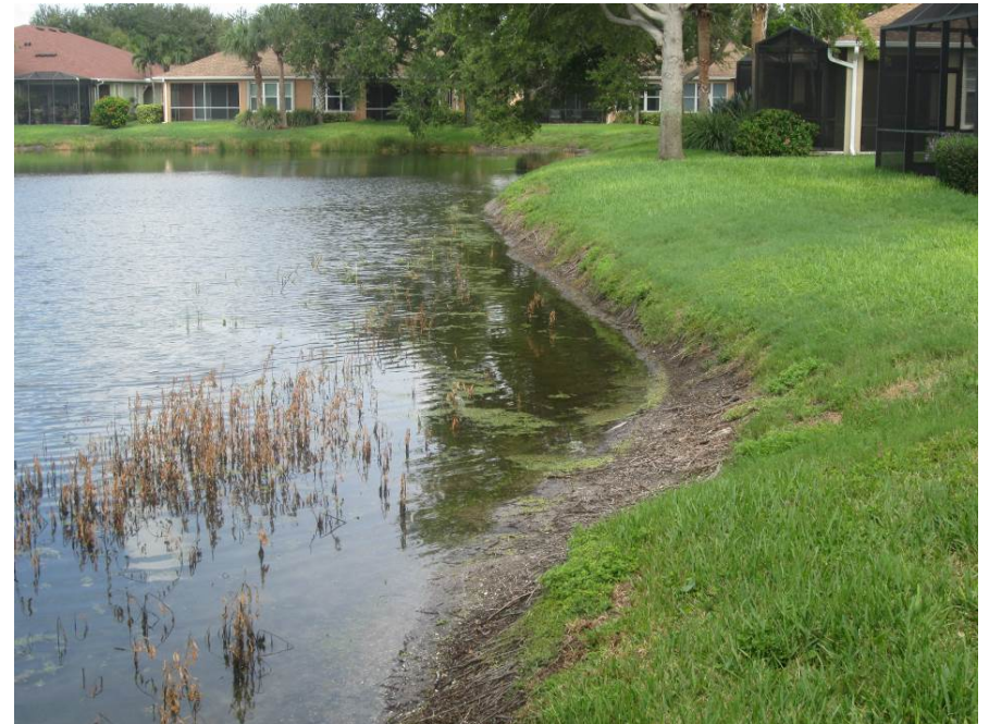
Pond 3 – 12"-18" of vertical erosion along north bank
