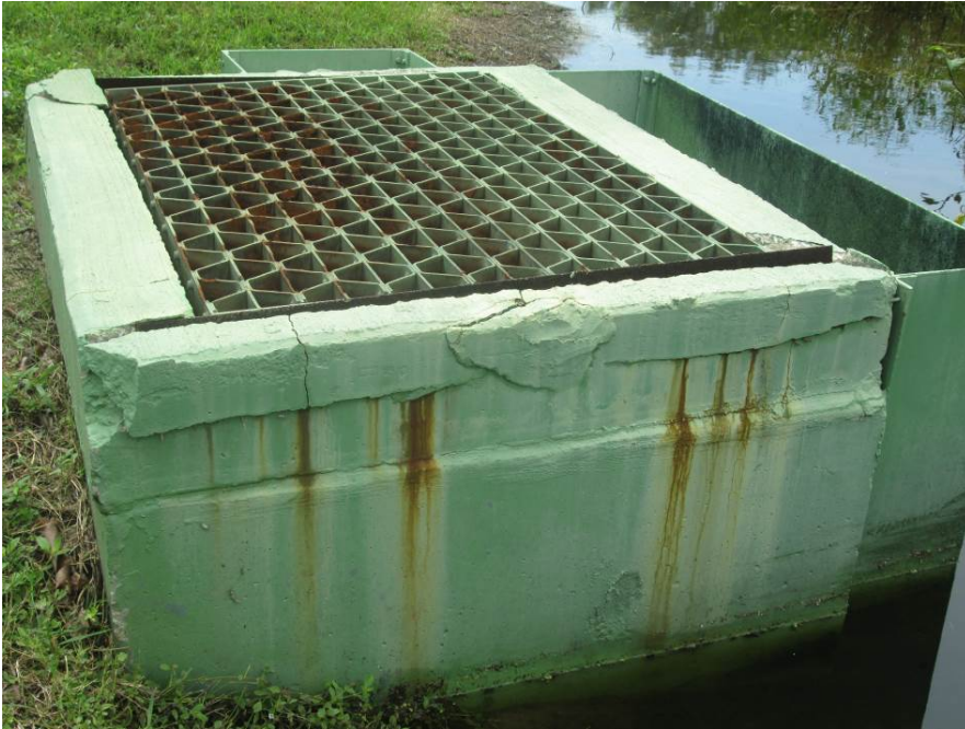
Pond 1 – Top of control structure cracked and needs repair
