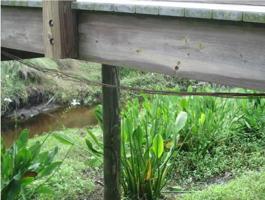
Wires hanging under southwest side of pedestrian bridge
