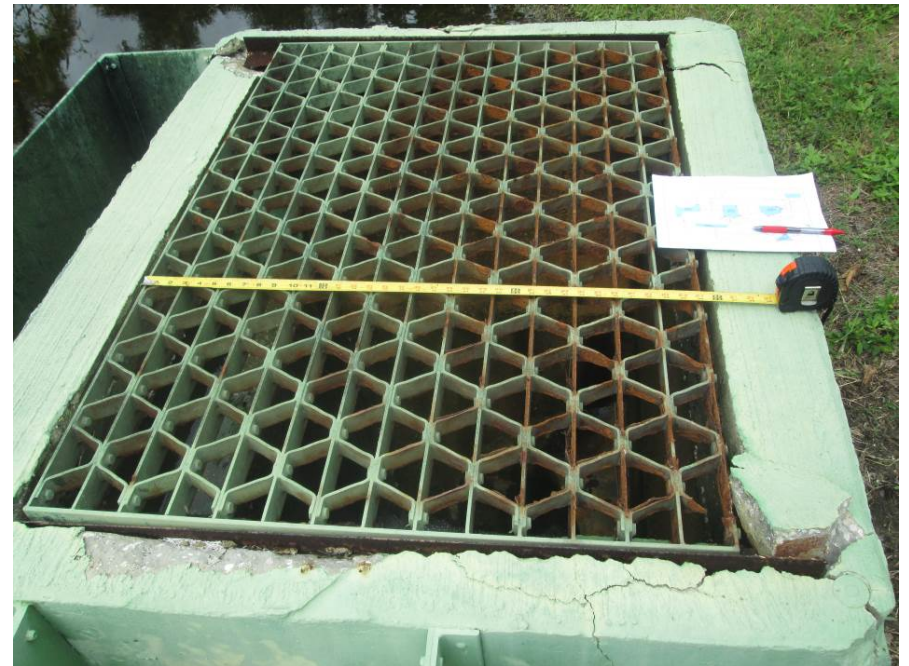
Pond 1 – Grate & frame rusting, should consider replacement soon
