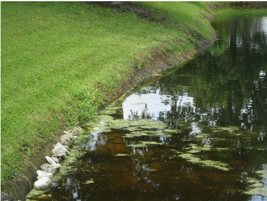
Pond 7 – Exposed geotube along east bank, add rip rap
