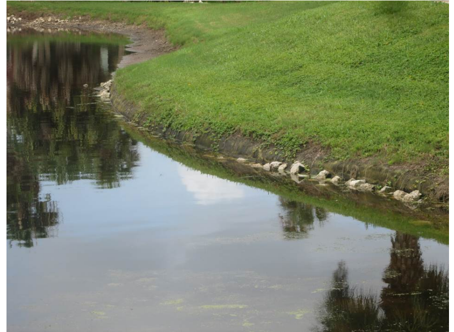
Pond 7 – Exposed geotube along west bank on south side, add rip rap
